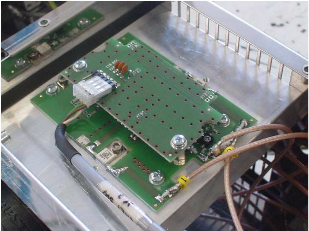
Exciter RF switch
